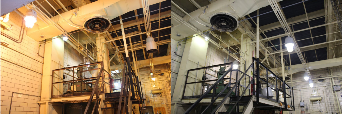
Before: 250W High Pressure Sodium Lamps
