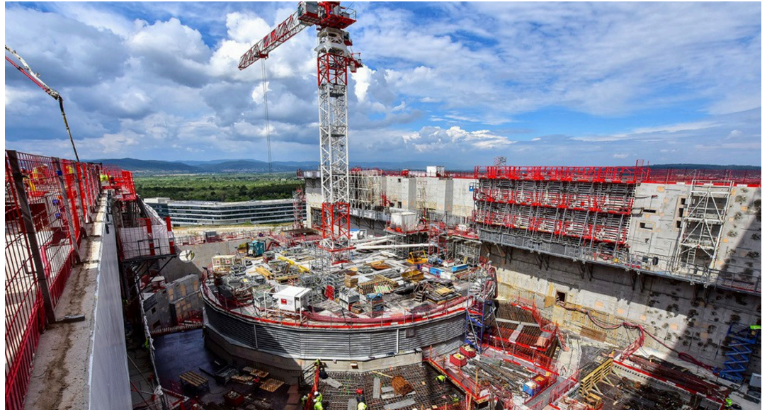
The tallest concrete of the Tokamak Building offers a spectacular and unusual viewpoint for works underway around the central Tokamak pit at the ITER construction site. © F4E
