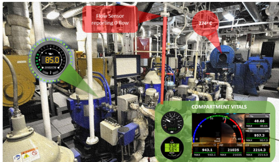
Figure 13: VR view (3D scan) of a ship compartment within the digital twin showing real-time sensor data overlay collected from the physical platform
