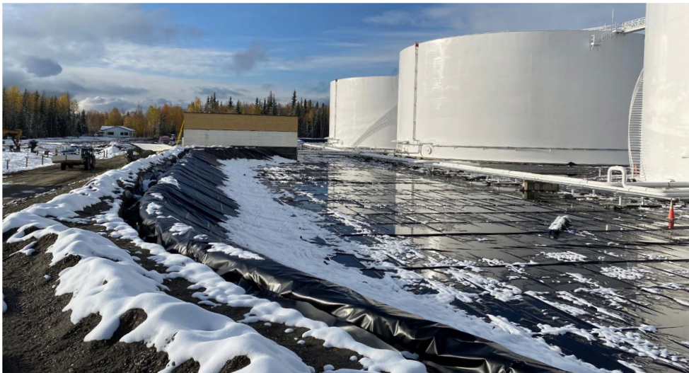
Figure 2 | XR-5 Ethylene Copolymer Geomembrane Lined Jet Fuel Secondary Containment Alaska, USA [photo source: Latitude 63 ]
